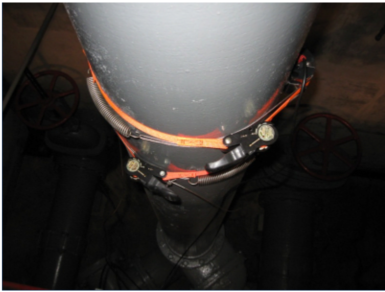
Flow meter 3, facing upstream
