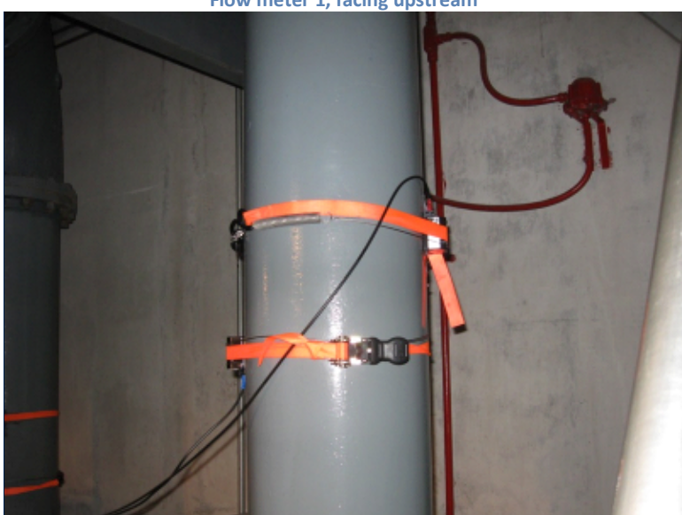
Flow meter 1, face
