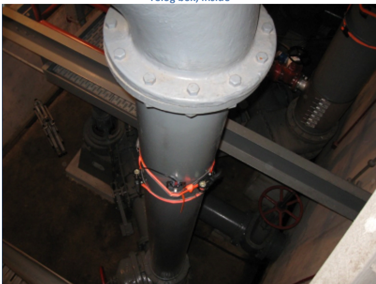
Flow meter 1, facing upstream
