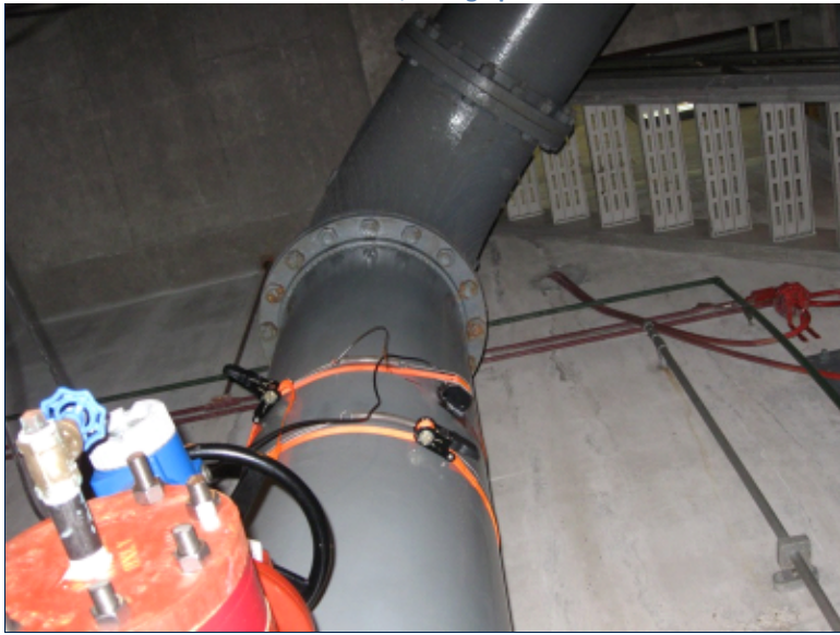
Flow meter 2, facing downstream
