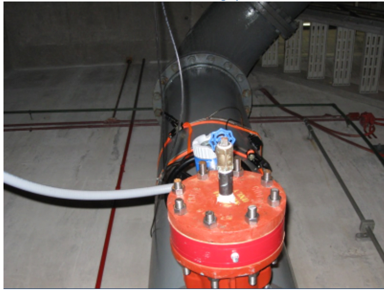
Pressure sensor, facing downstream
