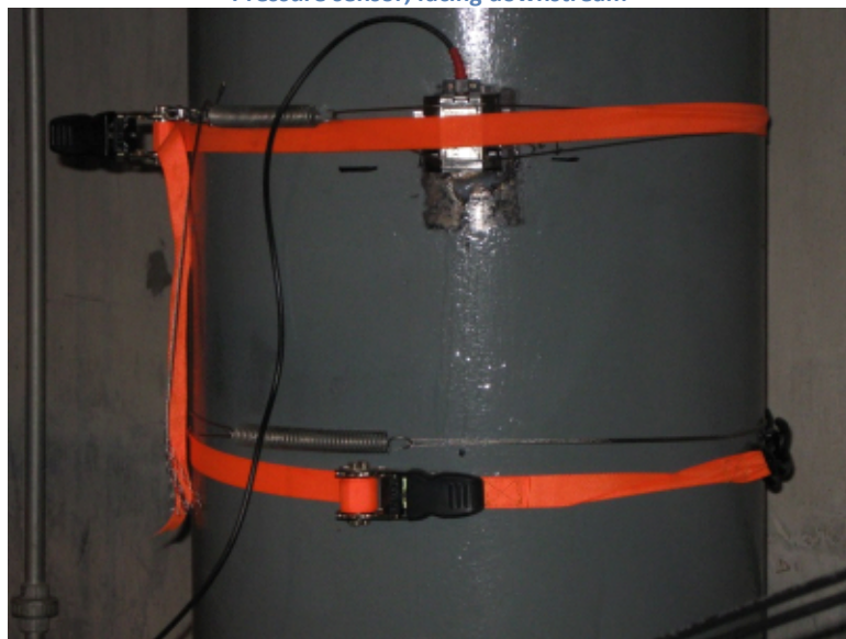
Flow meter 2, face
