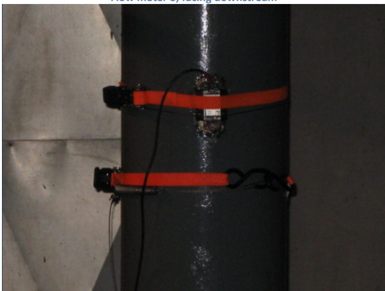
Flow meter 3, face
