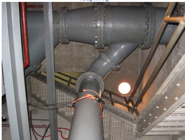
Flow meter 1, facing downstream
