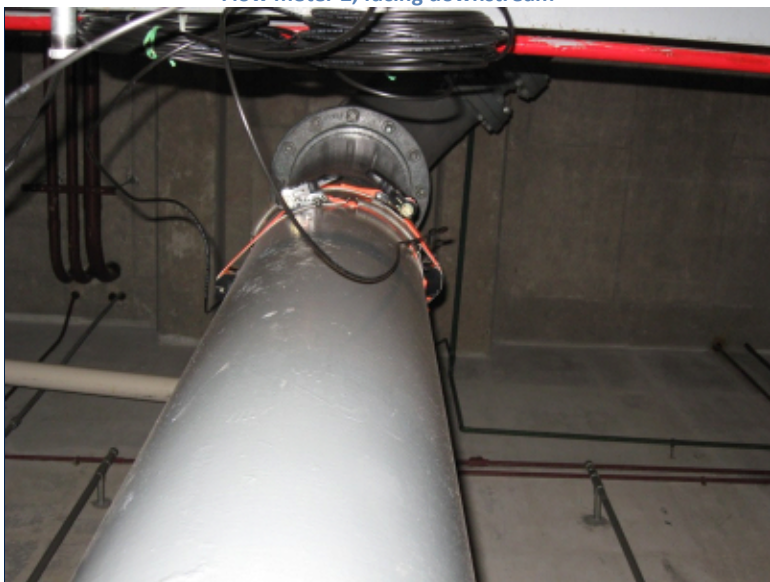
Flow meter 3, facing downstream
