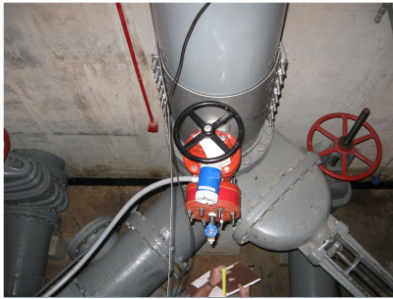
Pressure sensor, facing upstream
